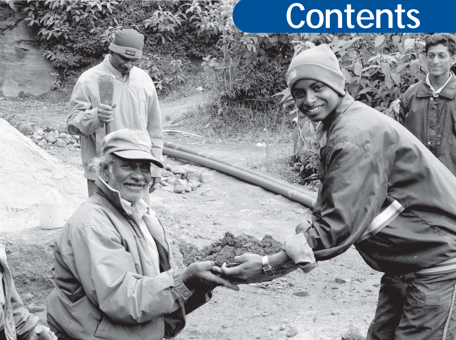
Above > Community members from Windicorner Village constructing a storage tank as part of the Community Water Supply and Sanitation Project.
